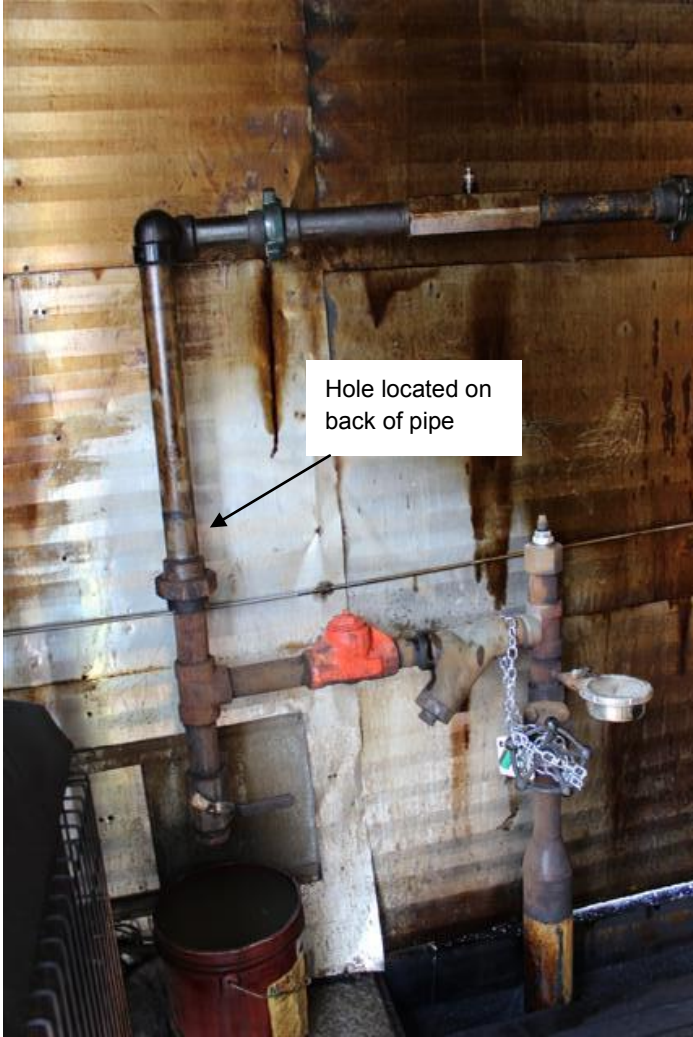
Figure 2. Lease piping prior to removal for analysis. (Source: AER)
