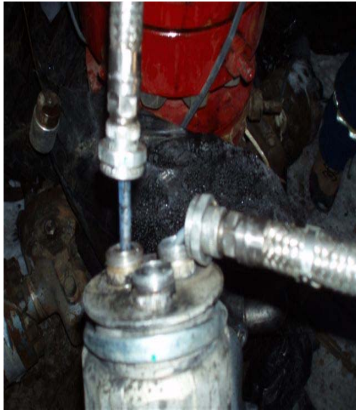
Figure 3a. Cable assembly detached at top of bracket assembly
