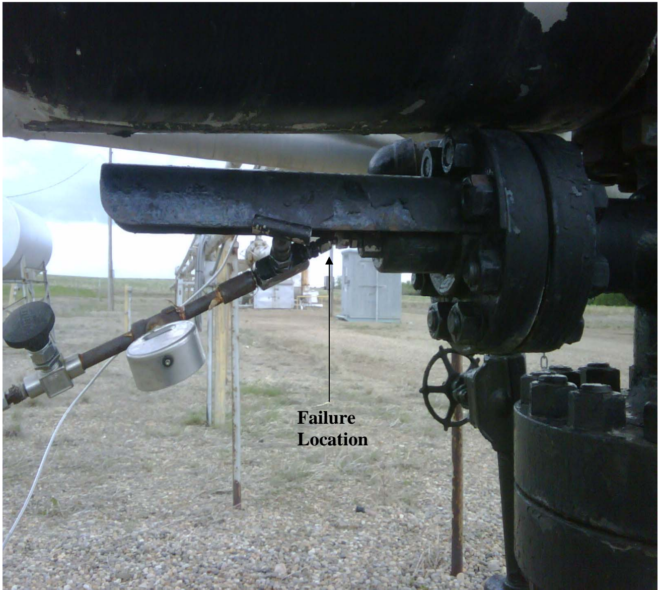
Figure 1. Failed hydraulic control line
